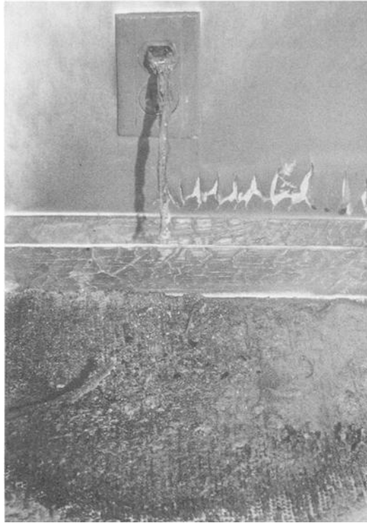
FIG. 3—A fire around a plug receptacle.
